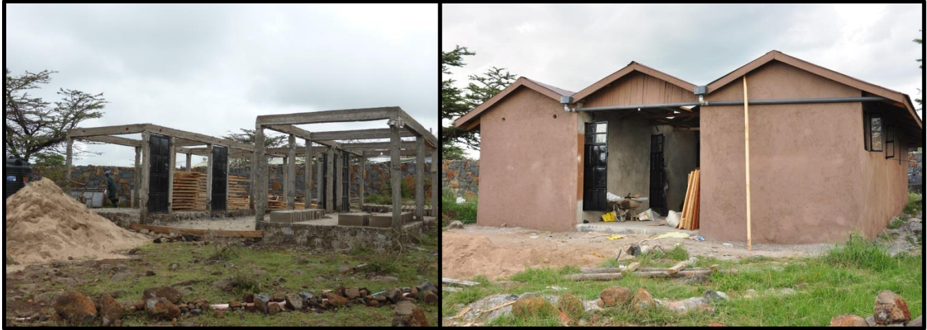
Figure 9: The upgrade of the Tony Lapham Predator Hub staff housing is almost complete! The photo on the left was taken at the end of March and the photo on the right was taken at the end of June.
